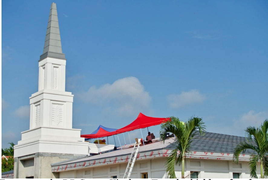
Figure 4. Tents atop the DR Congo Kinshasa Temple shield roofers from the sun. 26
